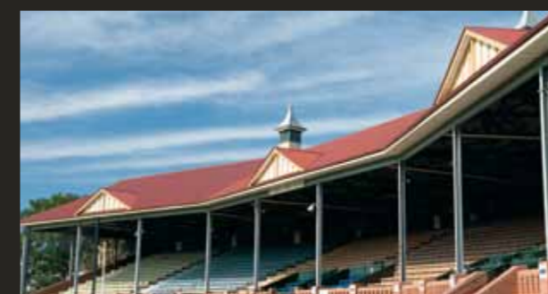
Norwood Oval's Grandstand retains its heritage with the new True Oak Deep profile.
